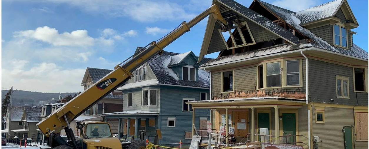
Figure 10: A material handler removes a panel of 206 College Avenue as it is being deconstructed. Photo by Felix Heisel, Circular Construction Lab
